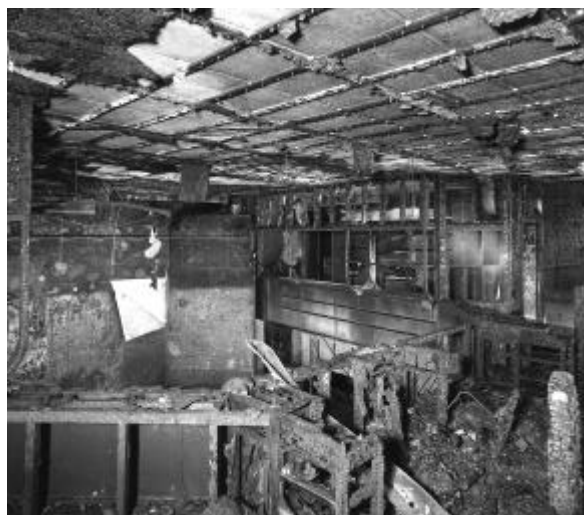
The burnt out operations room at Inverkip AAOR
